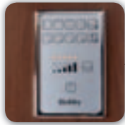
Central operating panel for lighting system and fresh-water level display
