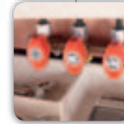
Central gas distributor in kitchen area
