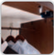
Wardrobe lighting with contact switch
